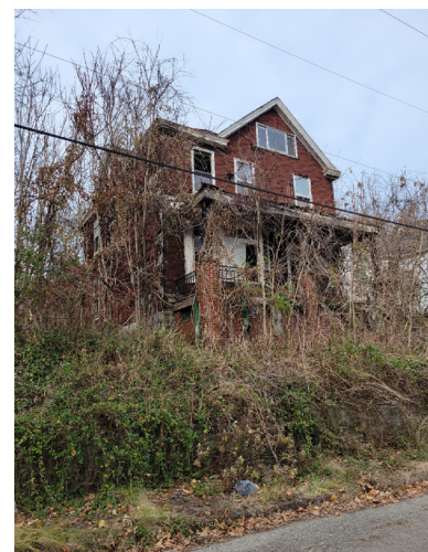
Blighted Property in Monessen Source: Westmoreland County Planning
