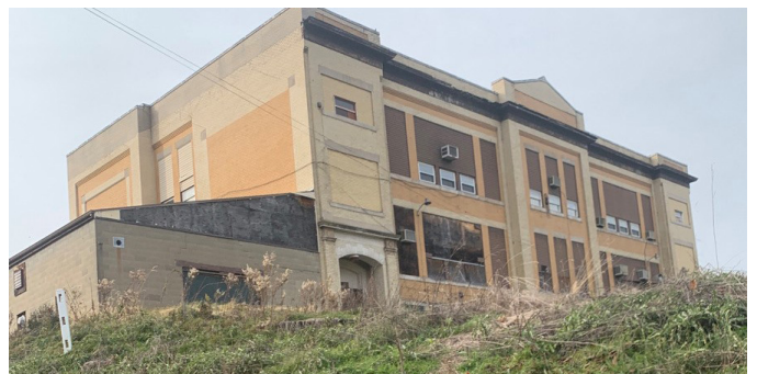
Blighted Structure in Monessen
